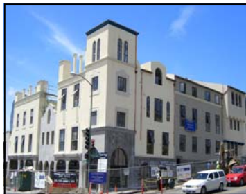
Piedmont Ave at Pleasant Valley, August 2007. Construction is due to be completed in September. Photo by Joyce Benna
